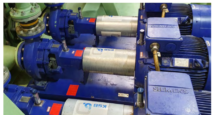
Figure 2. One unit of the water treatment installation, showing two wireless sensors on each pump.
