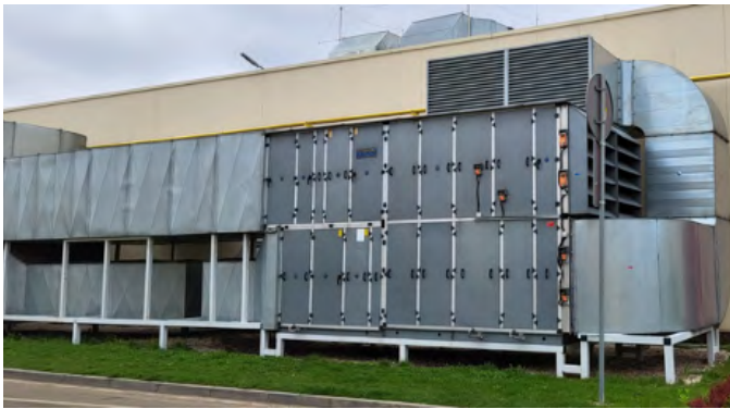
Figure 3. The critical air treatment system where 10 fans are monitored.
